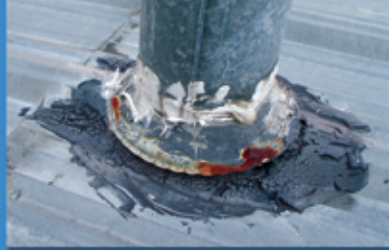
Damaged Vent Stack...
