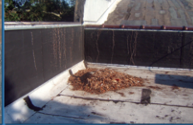
Debris Build Up...
